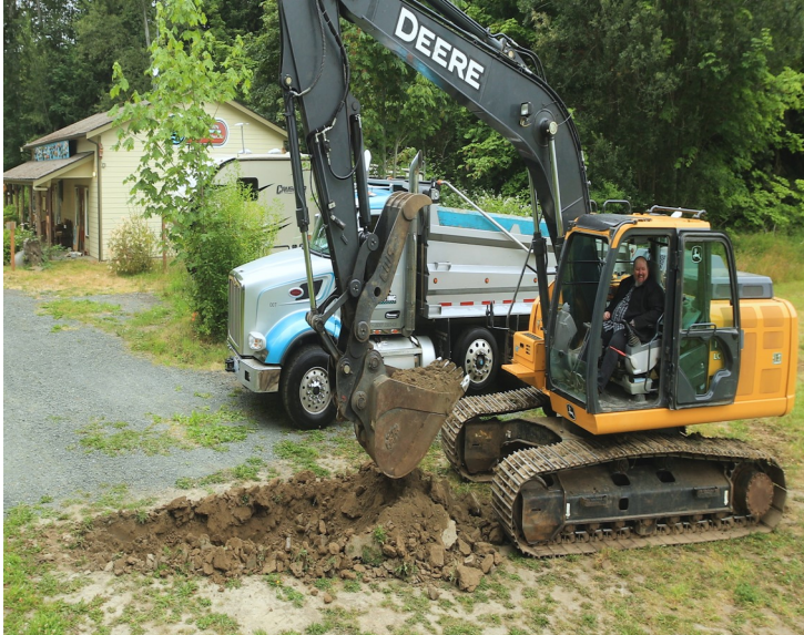
Breaking the ground by Kirk Nelson, Facilities and Construction Manager, Jamestown S’Klallam Tribe Photo by Silas Crews, Story Crane Productions
