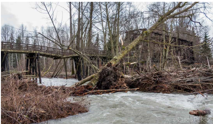
Damage to Railroad Bridge Trestle Photo by Chris Perry
